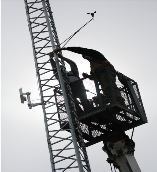
Wind directional and speed monitoring equipment being installed at the Dawson Creek Water Treatment Plant.
